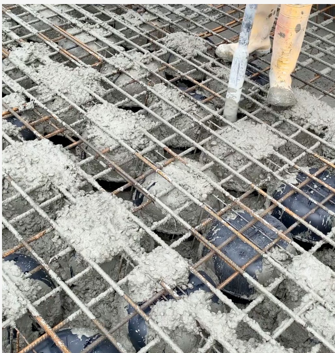
Concreting in two steps: First, the bottom reinforcement layer, to which the void former modules are attached, is concreted. Then the concreting of the slab is completed.
