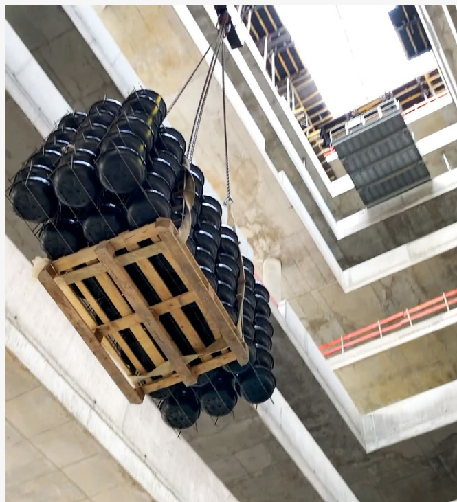
The void former modules are placed on the floor slab by crane and precisely laid by hand. Thanks to their low weight, only two people are needed for this activity. Source: Cobiax, Bielefeld.
